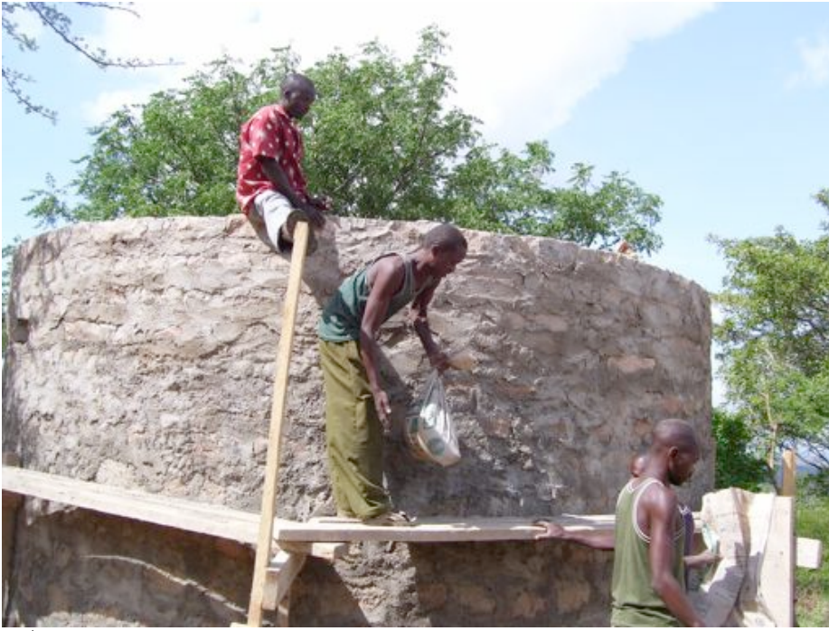
1 st collection tank which has already been completed and is holding water now
